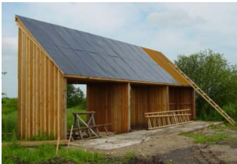
The solar kiln nears completion, awaiting the installation of fans and collectors this spring.
